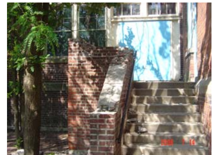
Deteriorated masonry stair prior to replacement.
