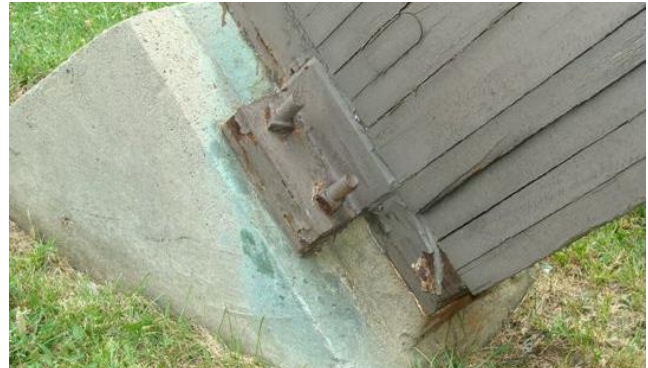
Deterioration of existing exterior glulam beam
