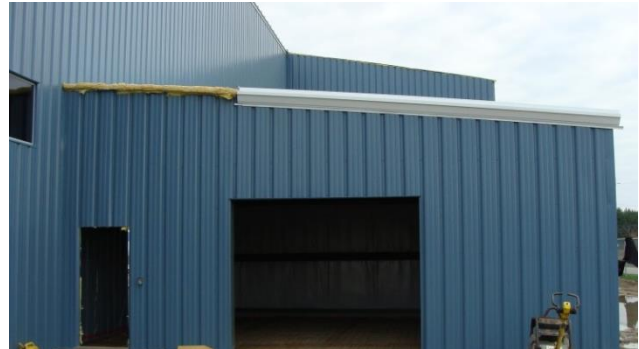
Ancillary building (30'x25') endwall elevation (roadside) with exterior cladding installation being completed
